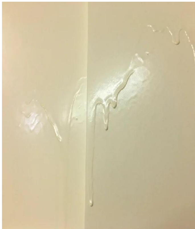
Figure 12: Unacceptable run / sag
